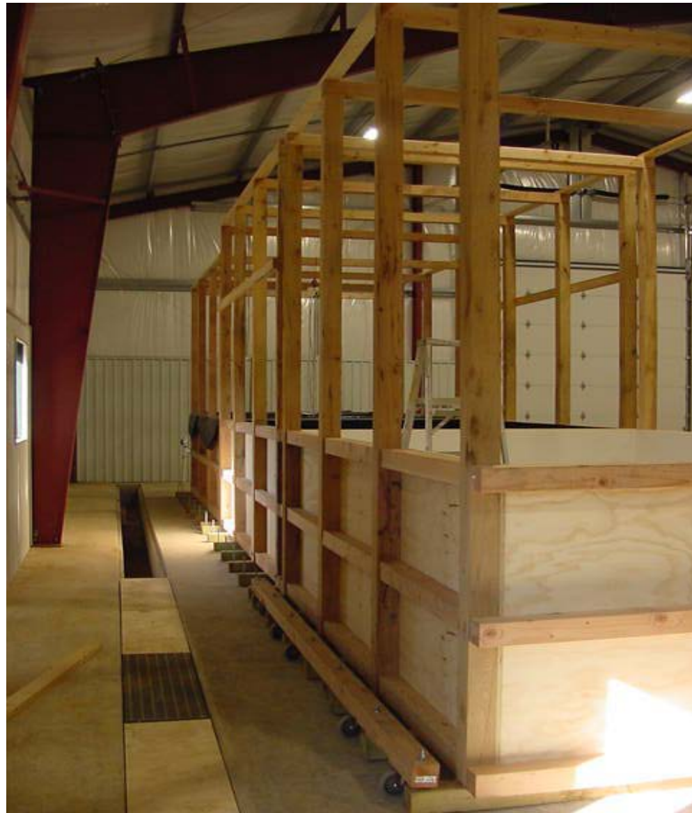
Prototype Raceways and Water Collection Sump
